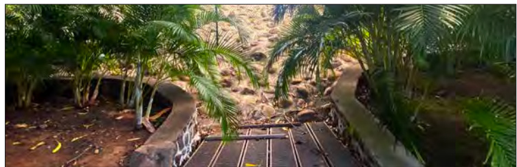
County repairs showing the new drainage system from Lower Honoapiilani Rd to the existing storm drain Source: Kahana Sunset photo archive (2023)
