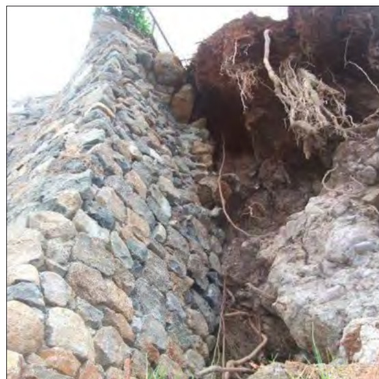
Photo of proposed repair area fronting A Building Source: AAA September 2009 File
