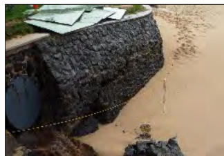
Storm drain prior to 2015 Source: Kahana Sunset photo archive (2011)
