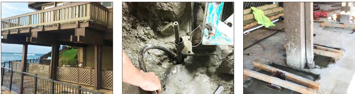
Process of installing micropiles to stabilize the A Building foundation Source: Structural Engineering Repair April 2018 File
