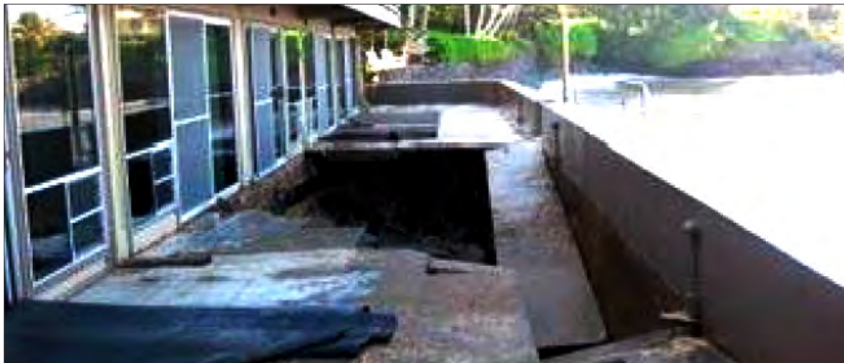
F Building sinkhole from December 2009
