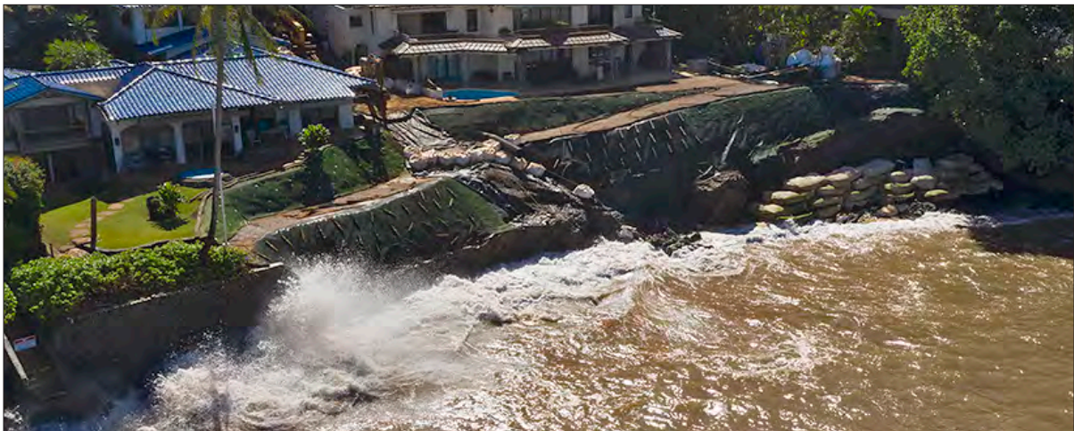
Seawall repairs made by neighboring properties during high wave surf event Source: Don McLeish January 2021
