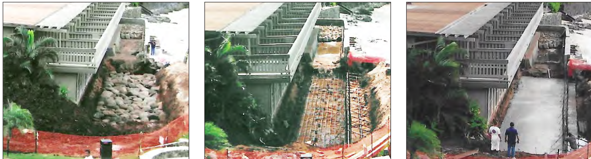
Workflow process repairing the F Building lanais Source: AAA Structural Engineering Repairs and Building 2010 File
