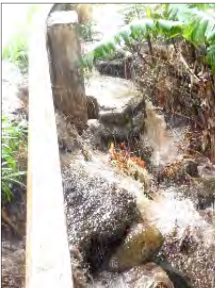
Flowing water from Lower Honoapiilani Rd into the storm drain Source: Kahana Sunset photo archive (2011)
