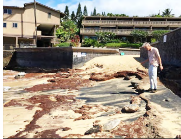
Exposed shoreline fronting the F Building and red clay 2016 Critical Impact Event Keonenui Bay
