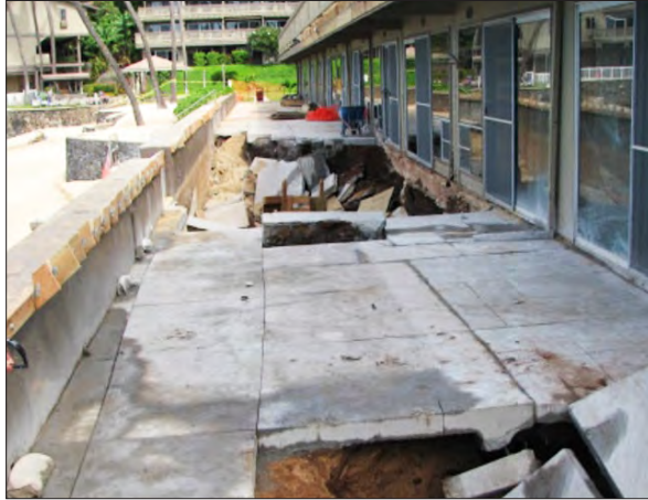
F Building lanais and sinkhole 2009 Critical Impact Event Keonenui Bay
