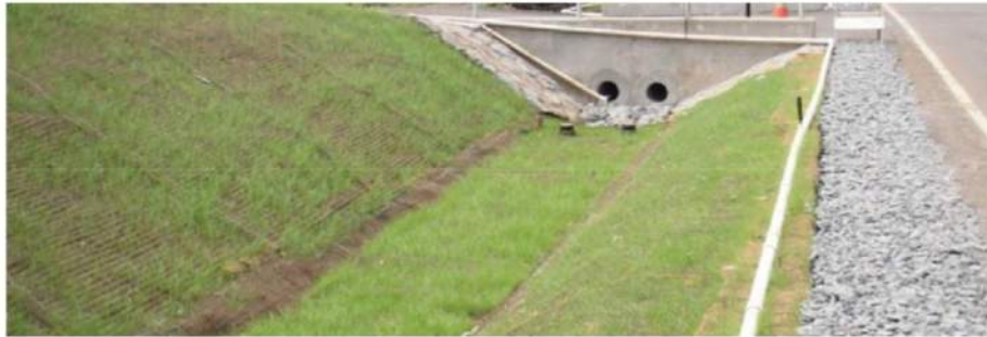
Bioswale adjacent to Kumuhao Street, Waimanalo, Oahu (Courtesy of the City and County of Honolulu)
