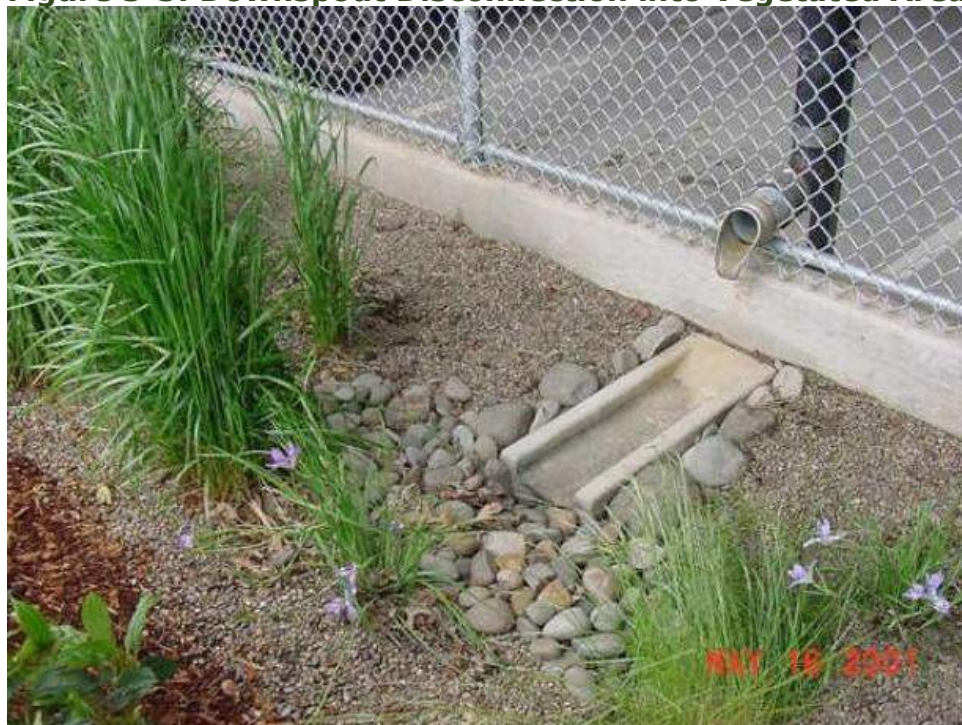
Figure 3-5: Downspout Disconnection into Vegetated Area
