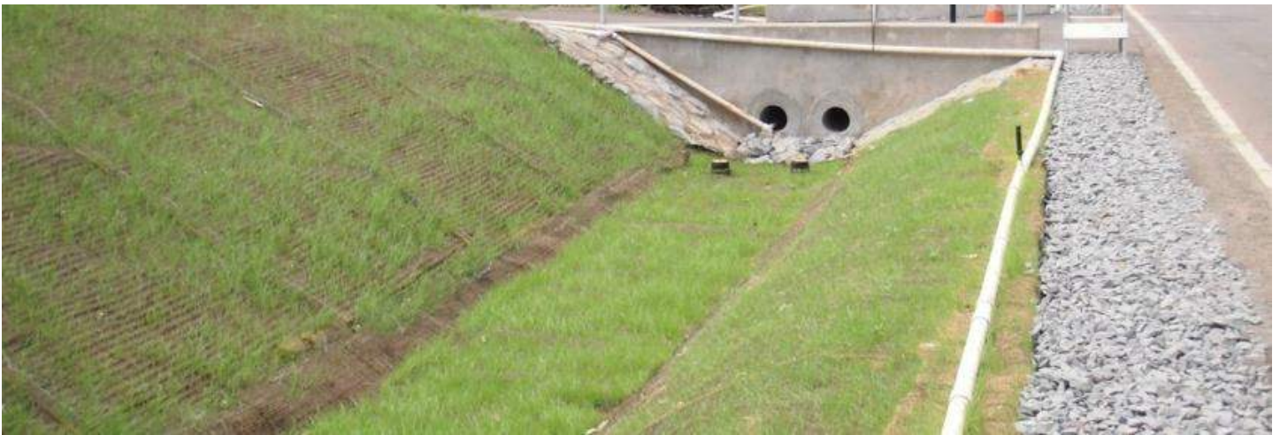
Bioswale adjacent to Kumuhaio Street, Waimanalo, O'ahu (Courtesy of the City and County of Honolulu)
