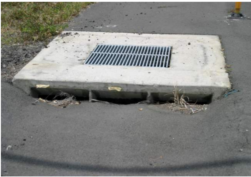
Dry Well on Ane Keohokalole Highway, Hawai'i Island (Courtesy of Bowers + Kubota Consulting)
