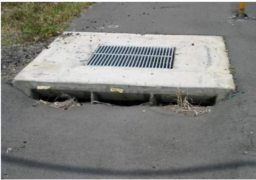
Dry Well on Ane Keohokalole Highway, Hawai'i Island (Courtesy of Bowers + Kubota Consulting)
