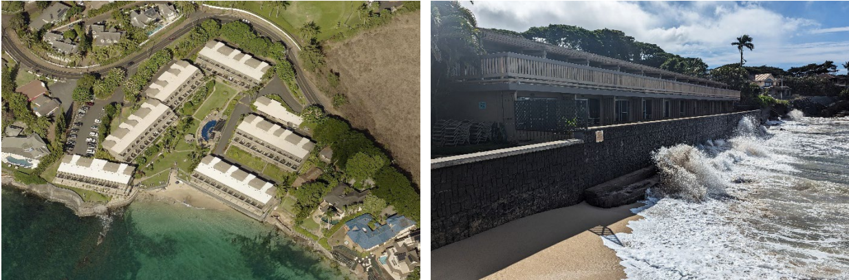
Kahana Sunset has experienced beach erosion that has rendered Building F uninhabitable, shown here in November 2023 (Photo credit L-R: EagleView CONNECTExplorer; SSFM)
