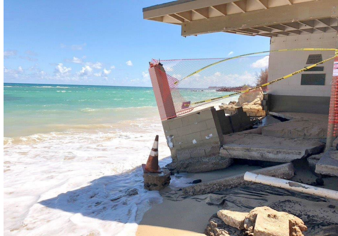
Damaged pavilion at Baldwin Beach Park, Maui following high surf in August 2020
