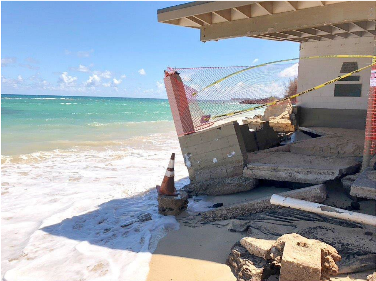
Damaged pavilion at Baldwin Beach Park, Maui
