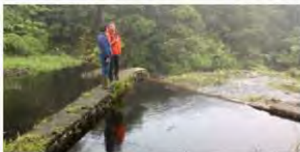
Hawai'i Department of Water Supply diversion intake (Marine Dam) on Waikoloa Stream.
