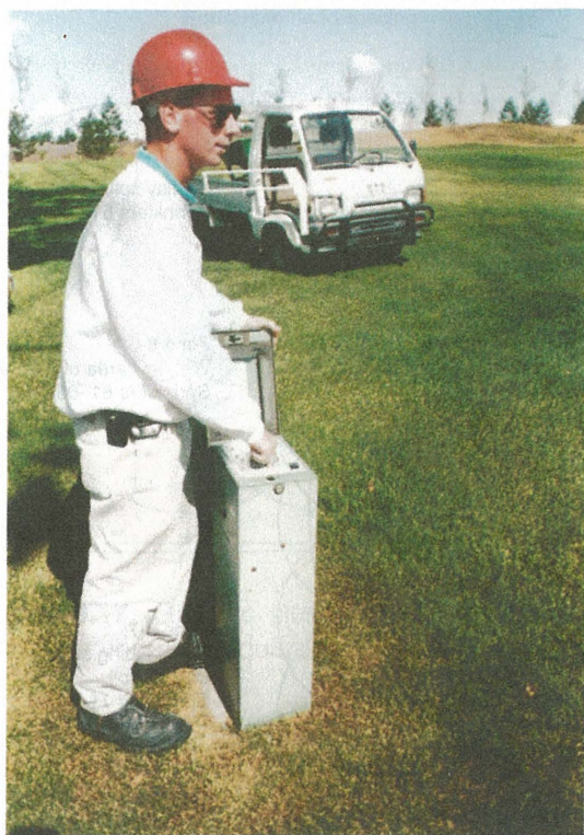
Figure 9.19. Satellite controller positioned so that it is possible to visually assess whether all sprinkler heads under its control are operating properly.
