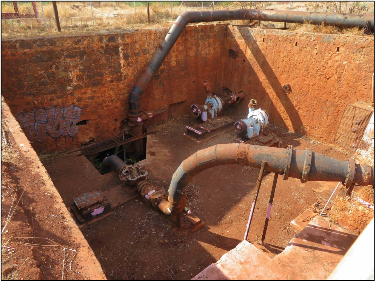
Within Shaft Pump House tunnel opening, note piping and old motors, looking directly Northwest
