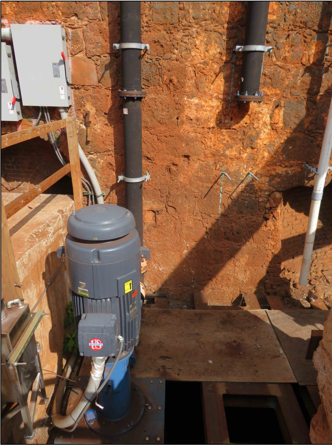
Within Shaft Pump House looking at motor, piping, and opening to water looking Directly East
