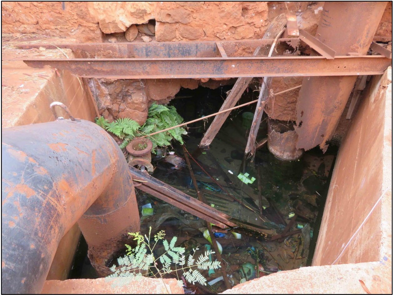
Within Shaft Pump House, tunnel with trash at west end looking directly Southwest
