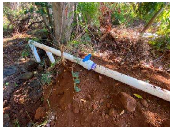
D) Newly installed end of lateral 4-inch line at drop point to South Waikapū Kuleana ‘Auwai considerably reduces water loss from Reservoir 1 nearly 1-mile upslope.
