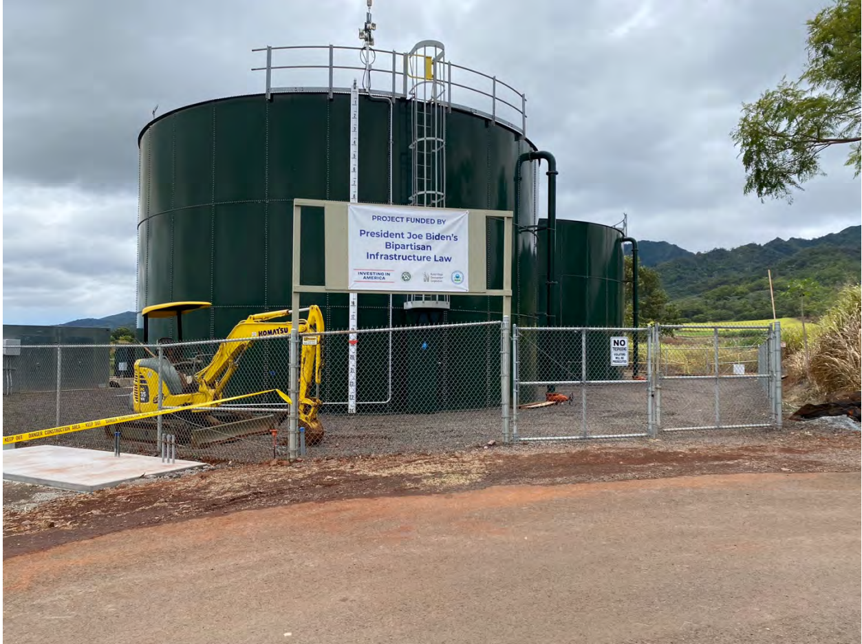
Looking southwest at the new water storage tanks where well will discharge
