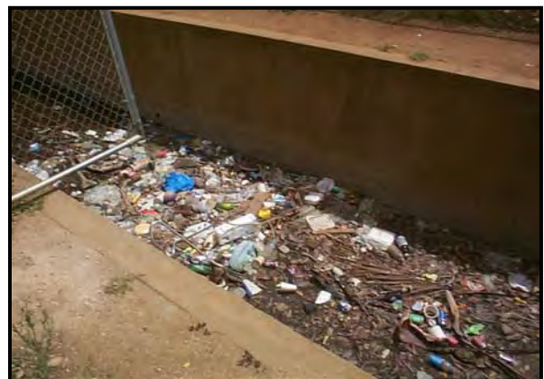
Trash in a Wai’anae drainage canal.
