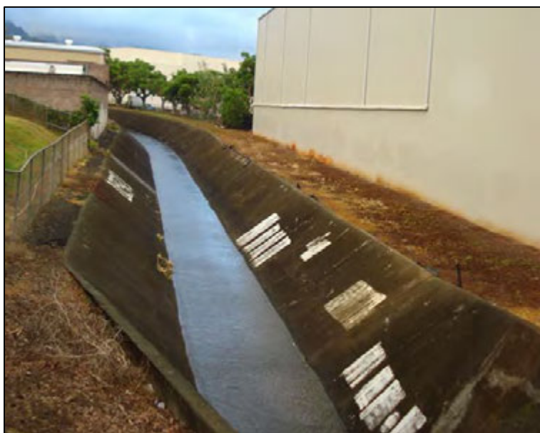
Kahuhipa Street storm drain
