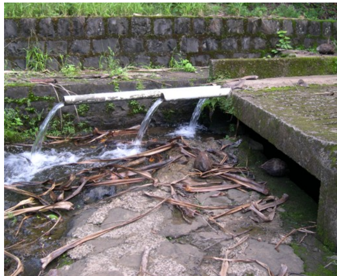
Bypass pipes at Haiku Ditch, Honopou Stream
