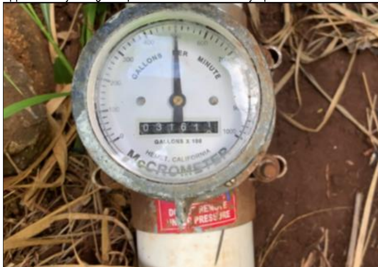
Photo 1. Wailuku Town Kuleana Pipeline distribution point meter showing approximately 500-gallon per minute flow with a fully-opened valve.
