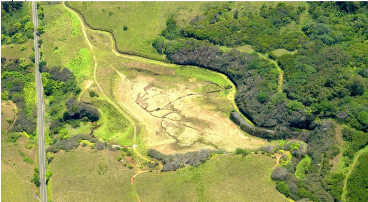
Figure 2: Site Photo, Kapala‘alaea Dam, looking east. Source: Hawaii DLNR Dam Inventory System; image date May 10, 2007
