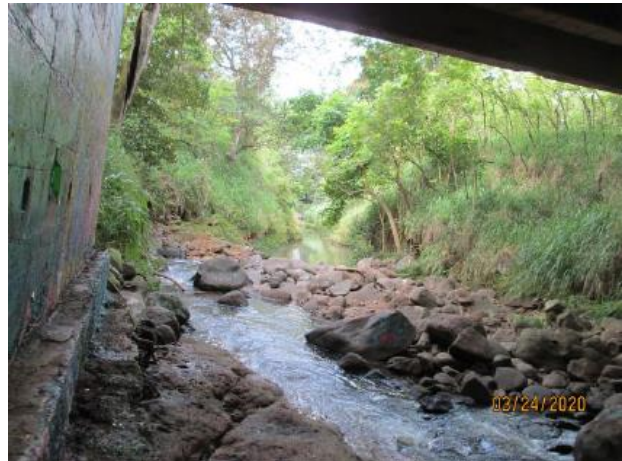
Looking downstream at location of DL 2 outlet and under Old Govt. Road Bridge.
