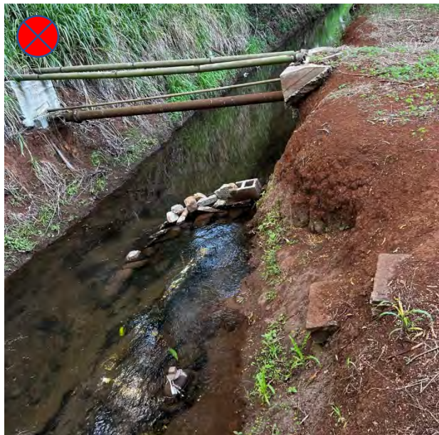
8-in kuleana pipe in Waihe'e Ditch that then enters Mundy's property.
