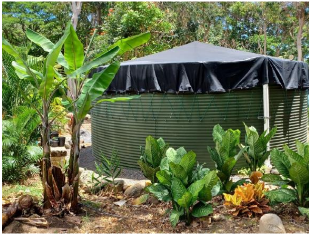
Rain catchment storage tank.
