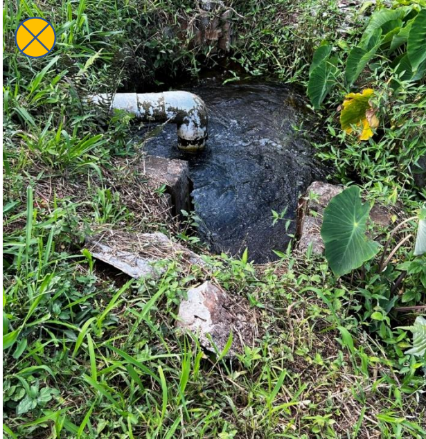
8-inch kuleana pipe at start of north and south side 'auwai.
