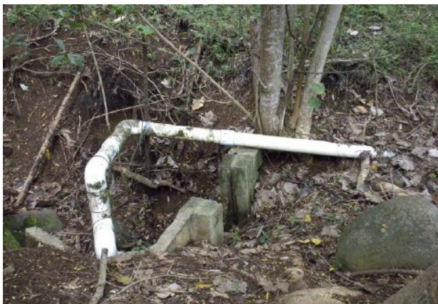
Wye joint basin – 4-inch "white pipe" turns north to Hoopii property.
