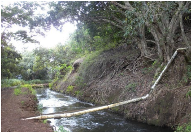
Start of 6-inch "white pipe" over Waihe'e Ditch. Shared source with Nakama.
