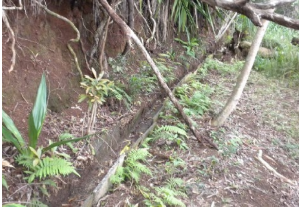
Cement flume carrying North Waiehu Stream water to "white pipe" over Waihe'e Ditch. Shared source with Nakama.
