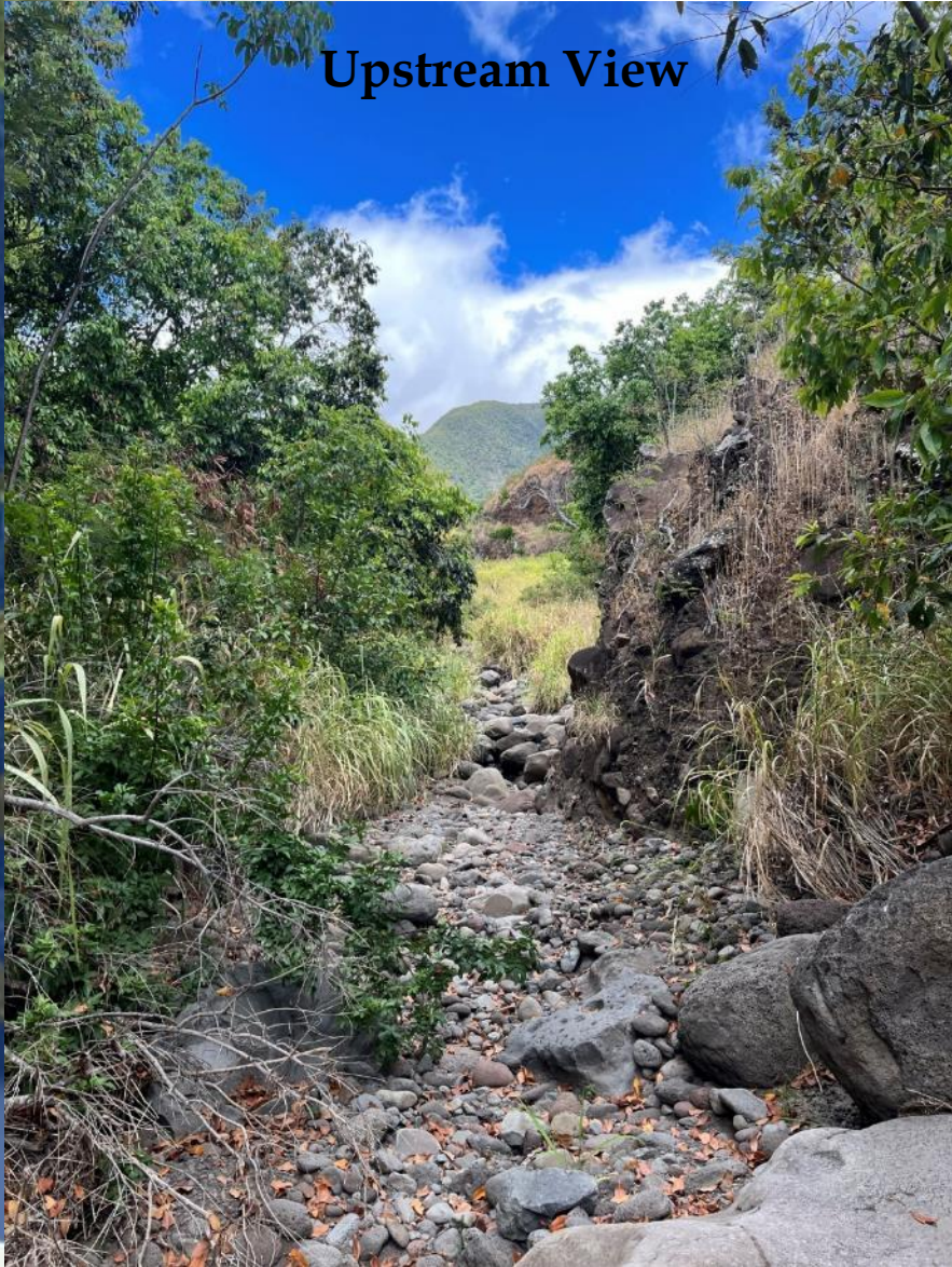
No flow at siphon
