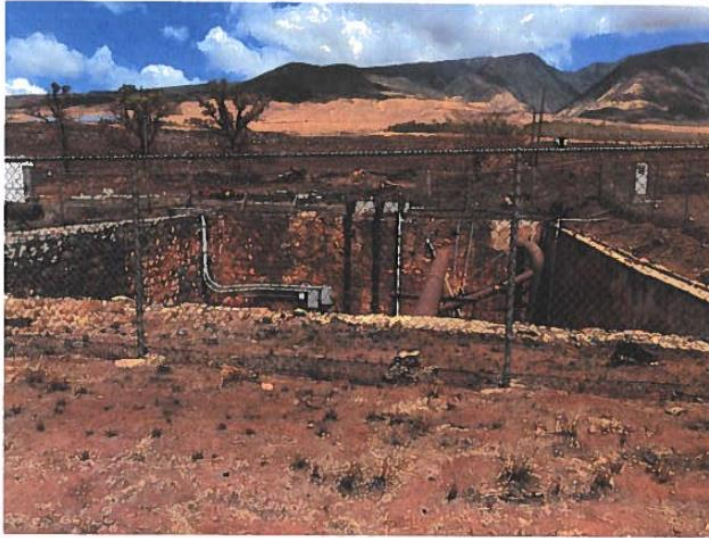
9 Well 6-5240-003 Pump A
