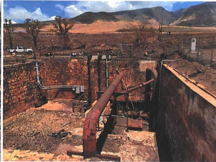
10 Well 6-5240-003 Pump A
