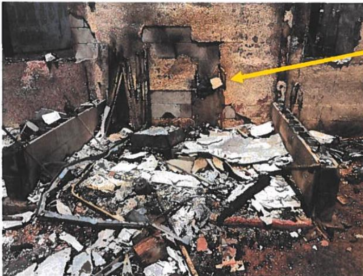
19 Well 6-5241-001: Lahaina Surf Bldg F Pump House
