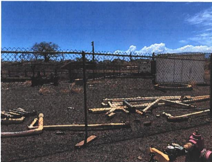
7 Well 6-5240-003 Pump A
