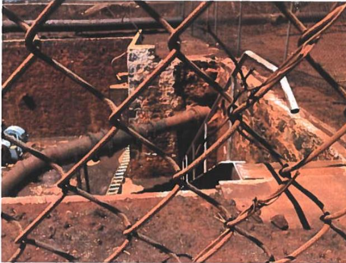
5 Well 6-5240-002 Pump B
