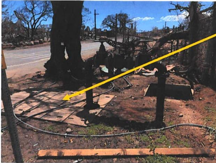
1 Well 6-5240-001: pipes at Lahainaluna Rd / Kahua St
