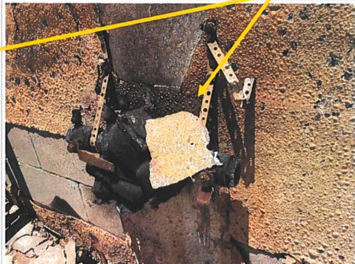
20 Well 6-5241-001: Lahaina Surf Bldg F pipes
