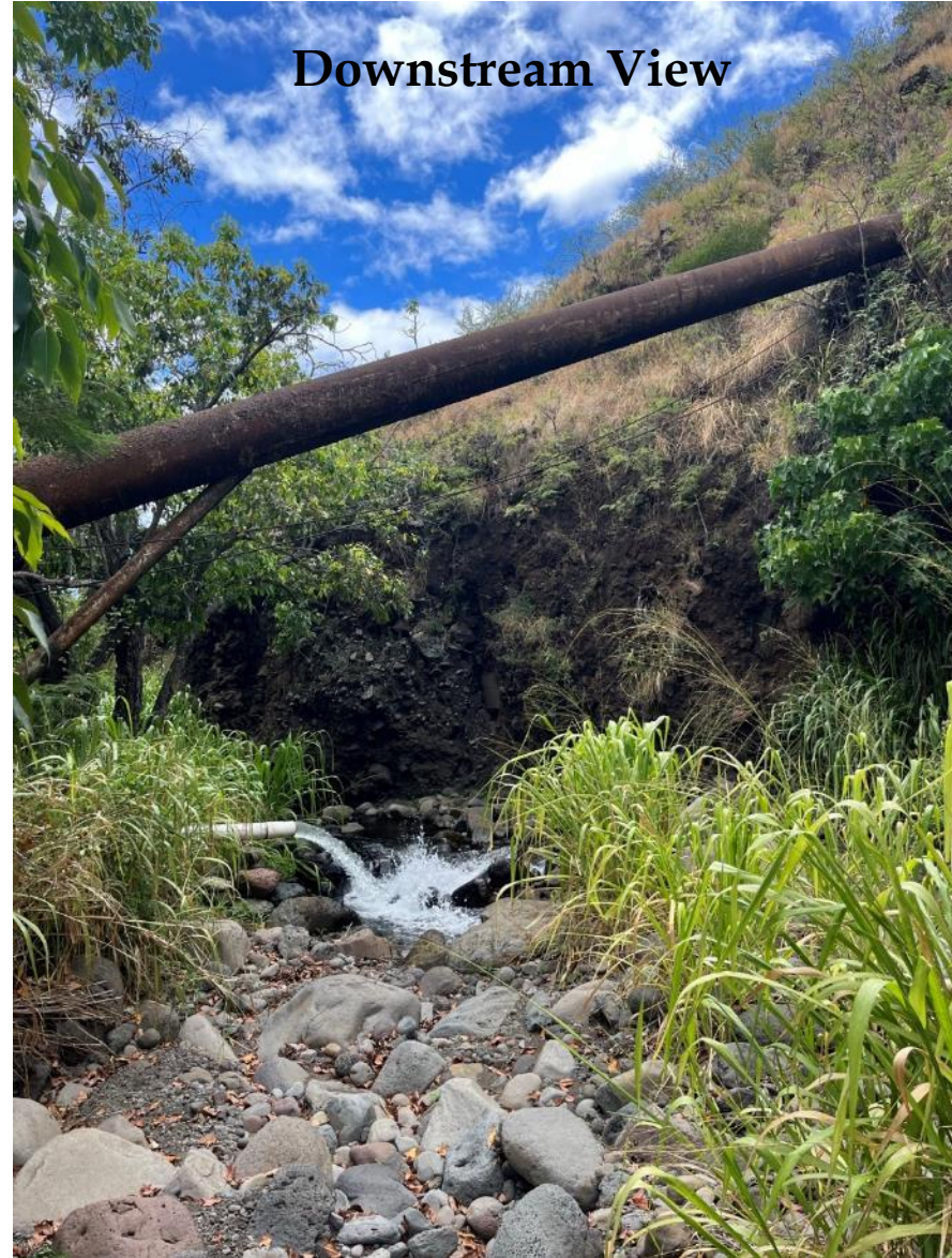
No flow at siphon
