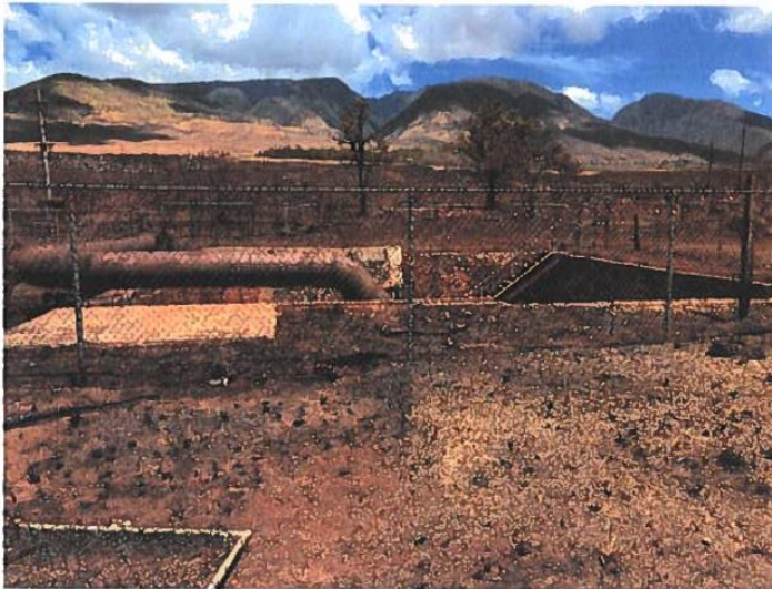
3 Well 6-5240-002 Pump B
