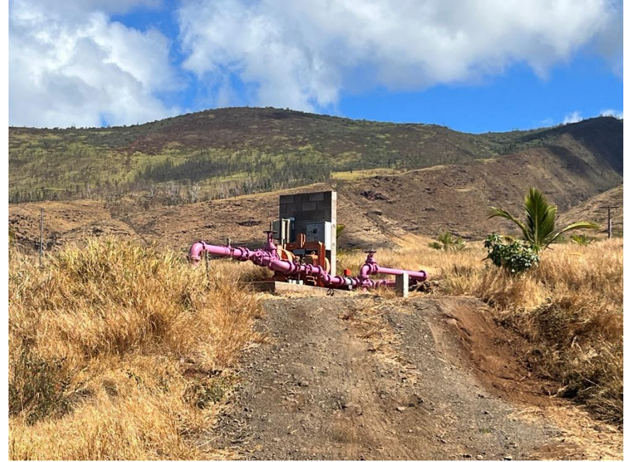
Kaua'ula Reservoir Booster Pump
