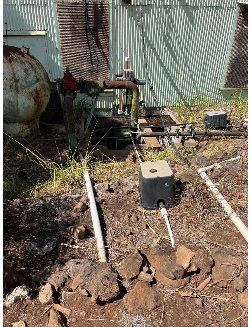
Kaua'ula Hydropower Penstock/Kapu pipelines
