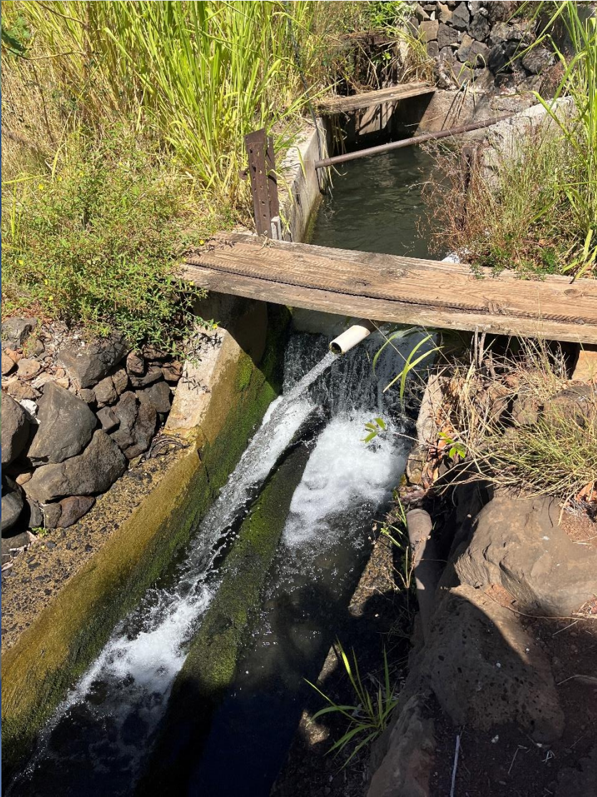
Kaua'ula Hydropower tailrace/Kuleana domestic pipeline
