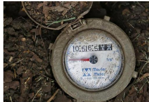
Customer meter under registration
