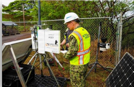
Air quality monitoring during tank degassing and ventilation
