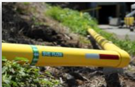
Soil vapor extraction and biodegradation studies to evaluate methods for site cleanup
