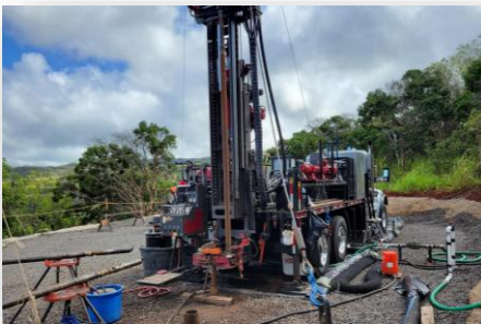
Expanding GW monitoring well network to increase visibility
