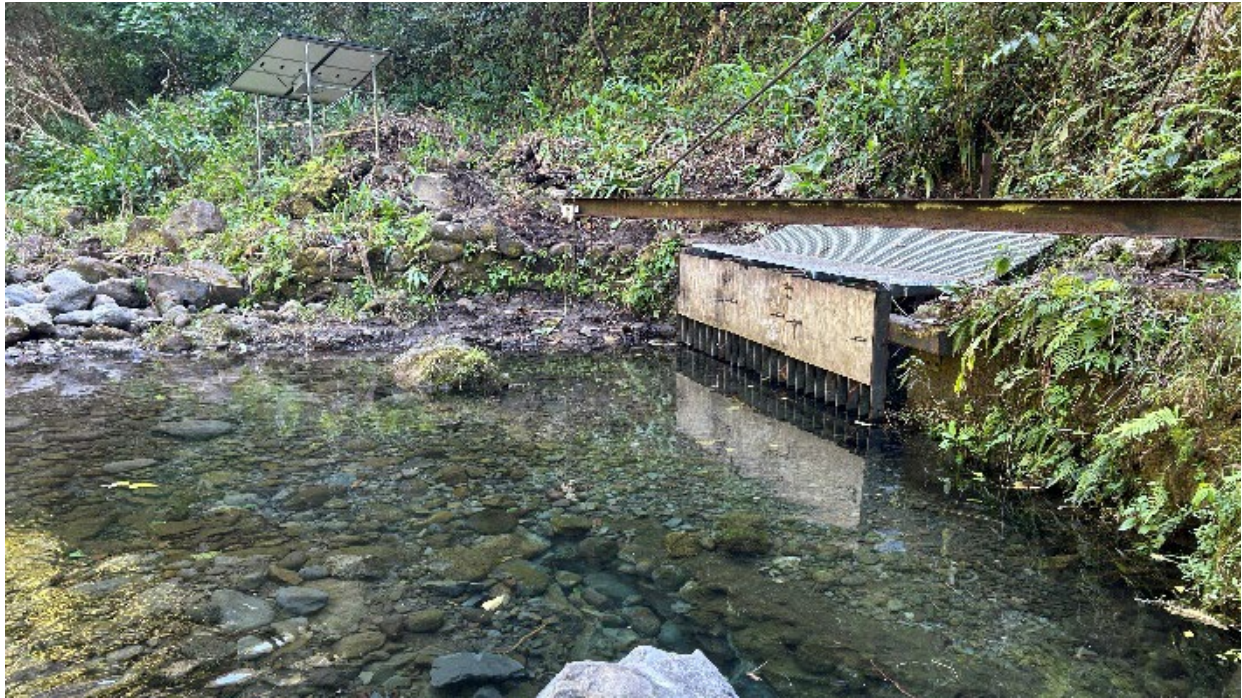
Figure 7. Close up view of trash rack on left bank at Diversion 770 (taken February 5, 2026).
