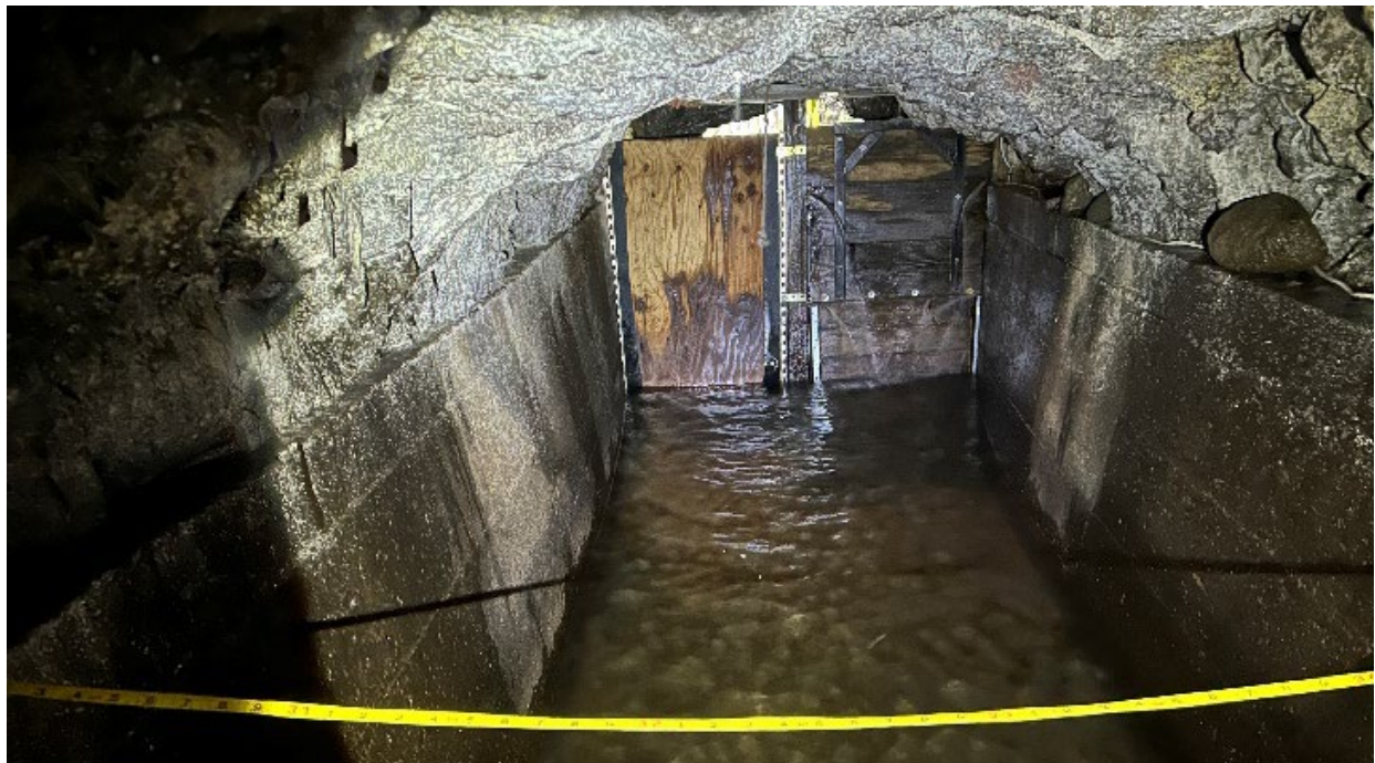
Figure 8. Upstream view of Diversion 770 intake at Aotaki Weir in Honokōhau Ditch (taken February 5, 2026).
