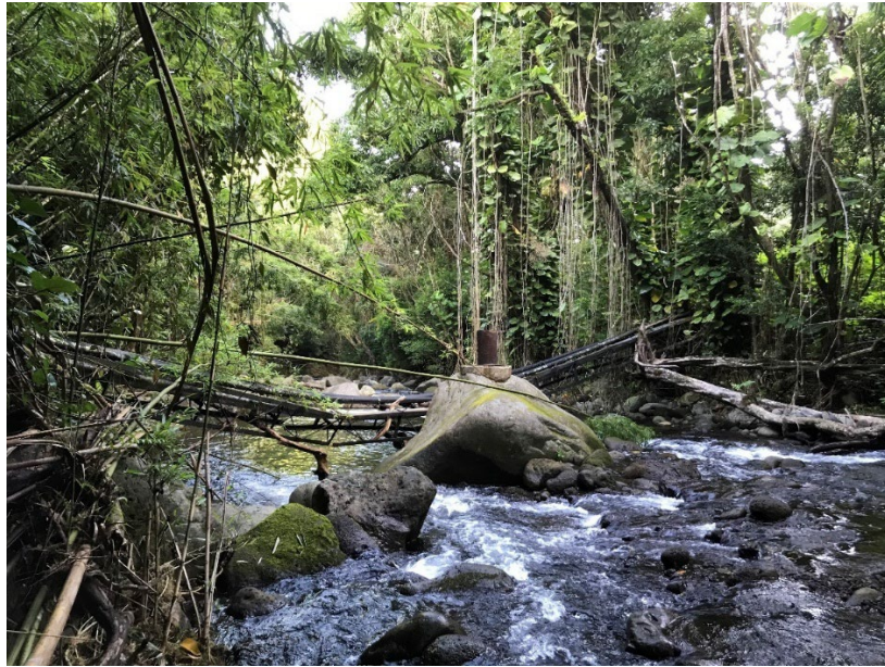
Figure 5: Image of the damaged bridge taken by Petitioner Eubank.
