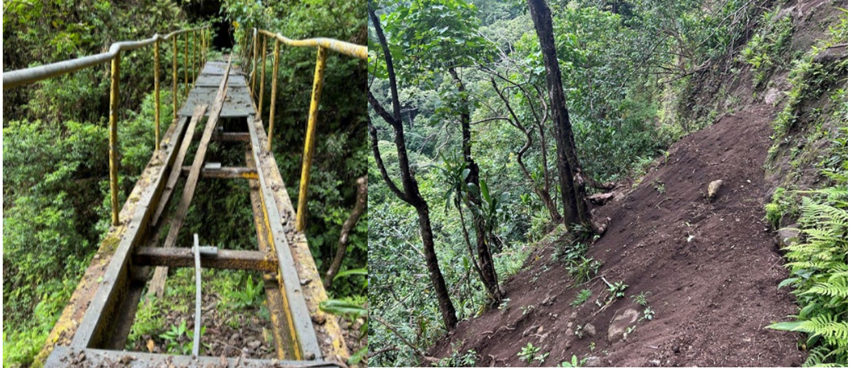
Figure 3: Images from the September 16, 2025, CWRM presentation shows disrepair of MLP’s Ditch System: Broken bridge used to access the Ditch System (left); Erosion on the trail used to access the Ditch System for maintenance (right). 64
