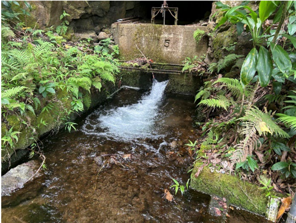
Figure 3. Picture of Adit 15 (Taro Gate) return flow from Honokōhau Ditch to Honokōhau Stream.
