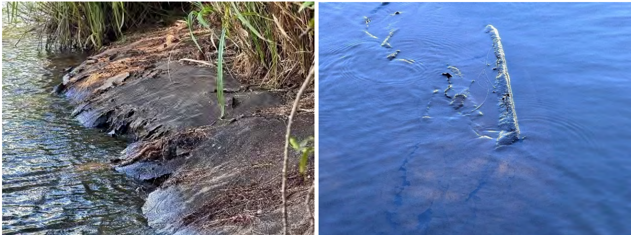
Figure 51: Severe deterioration of the liner of the Village Reservoir observed in July 2025. The photo on the left shows cracks in the liner visible from the banks of the reservoir. The photo on the right shows pieces of the liner that have detached from the bottom and floated to the surface.
