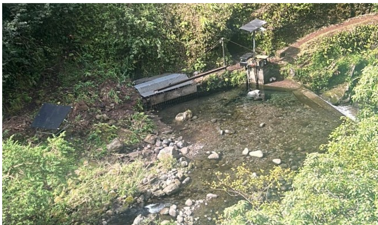
Figure 6. Aerial view of Diversion 770 with intake located on left bank (taken February 5, 2026).
