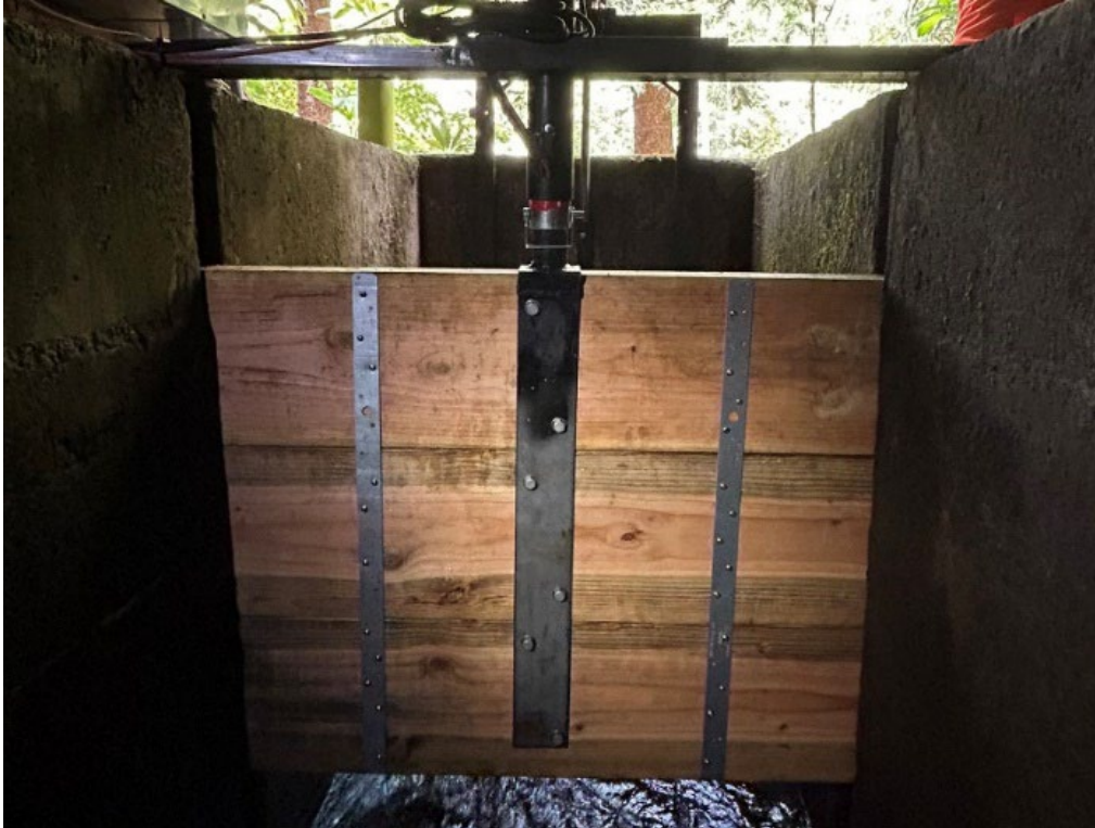
Figure 4. Remotely operable gate installed downstream of Adit 15 in Honokōhau Ditch to increase returned flow, June 14, 2025.
