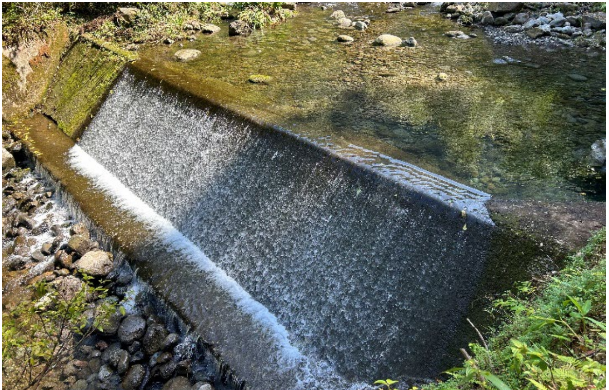
Figure 10. Aotaki Weir at Honokōhau Stream (taken February 5, 2026).
