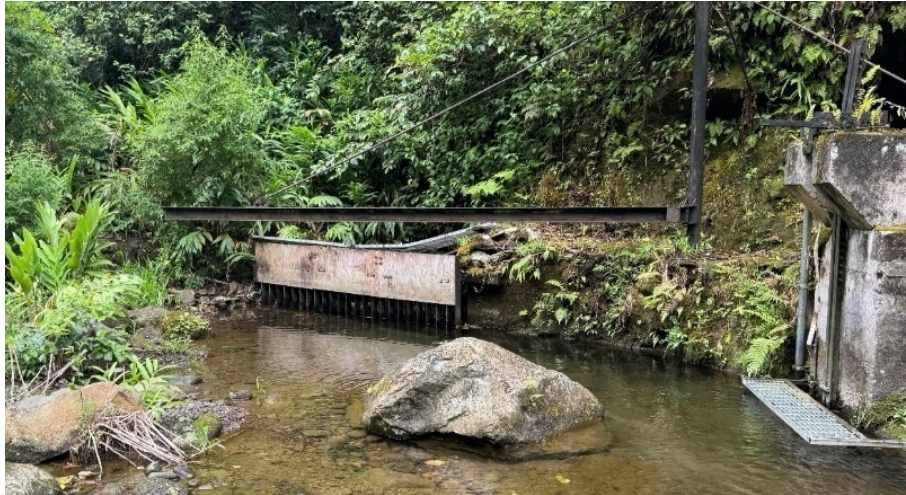
Figure 1: A photo from May 23, 2025, of the supposedly “temporary” plywood restrictor plate at Diversion 770 that CWRM allowed MLP to install in lieu of a remotely operated gate in 2021. This gate is allegedly being replaced by a remotely operated gate—a fix that MLP previously claimed was “impractical.”
