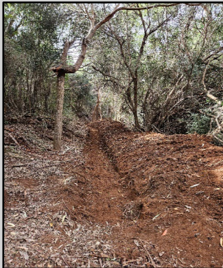
The bypass ditch is unlined and hydraulically inefficient.
