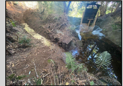
The inlet/bypass gates are essential to reservoir and ditch operations during low-flow periods, but are in disrepair
