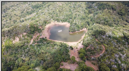
The water level in and releases from Pu'u Lua reservoir cannot be controlled because the discharge valve is inoperable.
