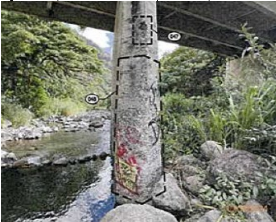
Figure 2b: A photo of abrasion on a pier to be repaired.
