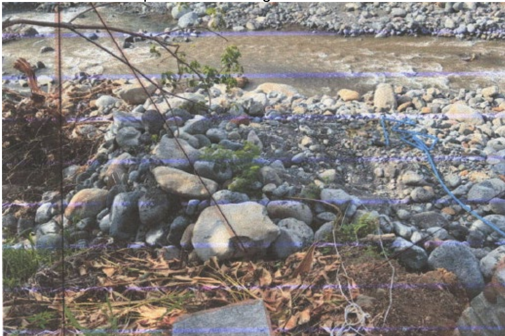
Figure 4. View from top of left streambank. A portion of the concrete stairs that washed away is visible in the bottom right of photo. Rocks were piled against the denuded left bank to reach the top of the remaining stairs.
