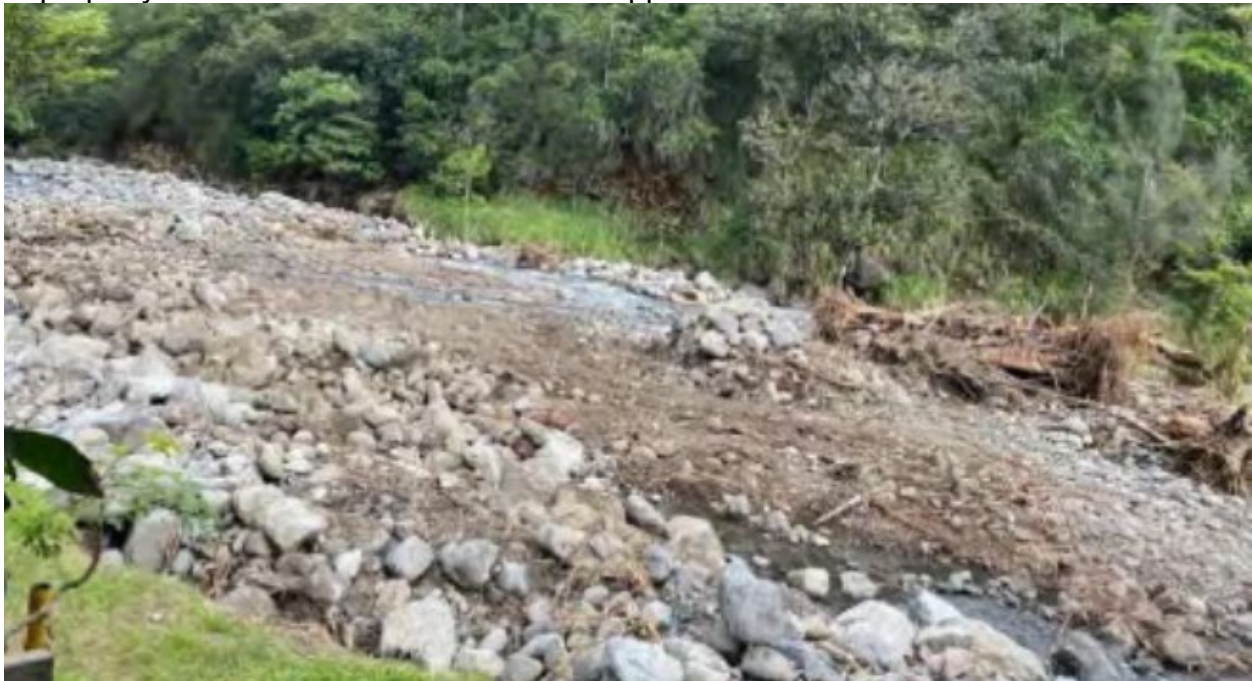
Figure 4. View from right bank of river with rock berm created in the foreground at edge of property to divert streamflow toward the opposite left bank.
