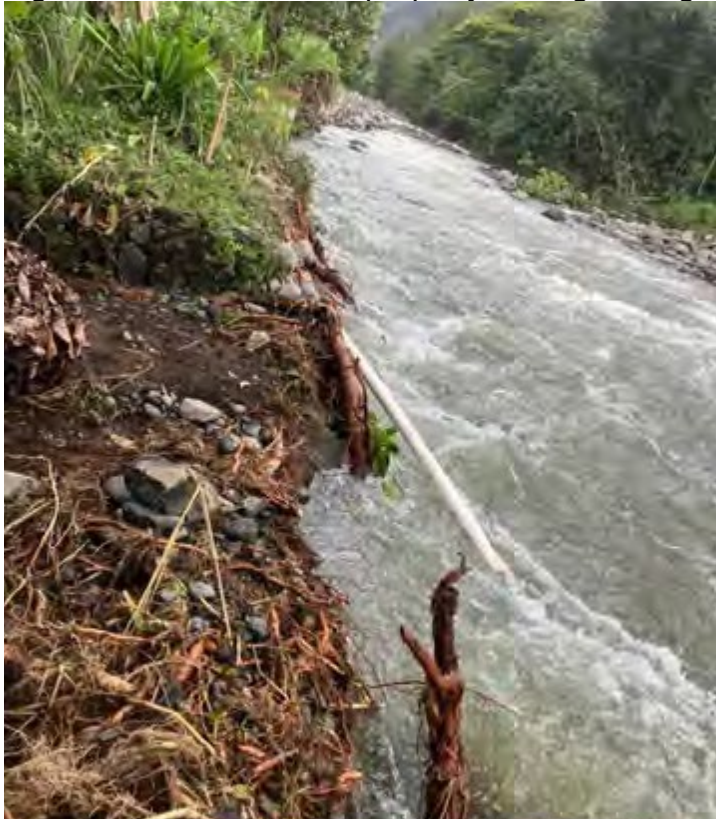
Figure 2. View of Gomes property damage on right bank of stream, looking upstream.
