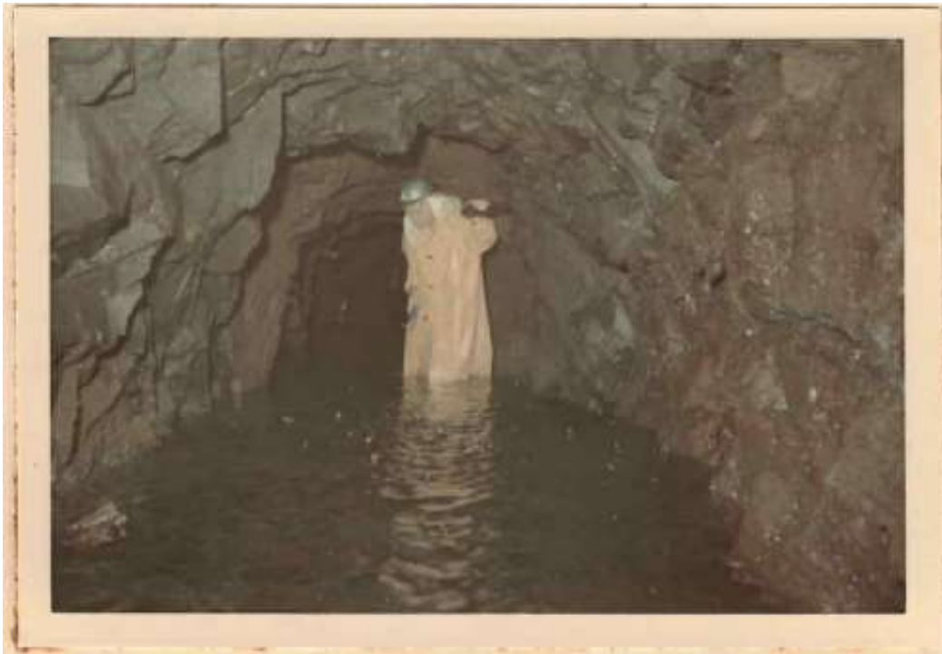
Figure 7: “View looking towards portal at about 1000-feet in Ha’ikū Tunnel showing saturated rock in foreground and dike at STA 9+80”. (Bowles, 1969)
