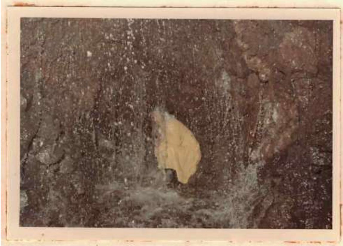
Figure 10: “View of Ha’ikū Tunnel heading, majority of discharge is from drill holes in clinker” (Photograph from Bowles, 1969)
