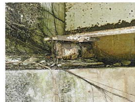
3 PHOTO - ROLLER BEARING CORROSION AT IAO ABUTMENT NOT TO SCALE
