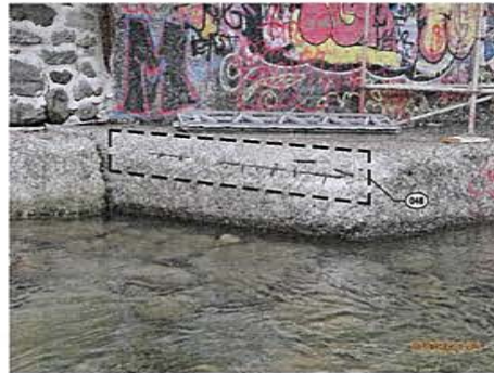
5 PHOTO - SPALL ON ABUTMENT FOOTING NOT TO SCALE
