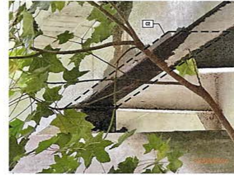
3 PHOTO - GIRDER CORROSION AT WAILUKU PIER NOT TO SCALE
