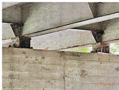
2 PHOTO - FIXED BEARING CORROSION AT WAILUKU PIER NOT TO SCALE
