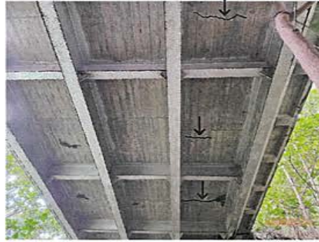
2 PHOTO - CRACKS IN DECK SOFFIT NOT TO SCALE
