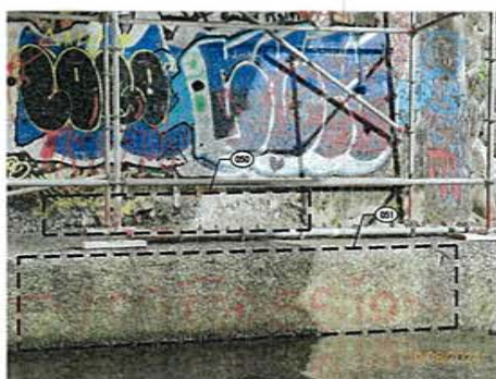
4 PHOTO - SPALLS / ABRASION ON IAO ABUTMENT NOT TO SCALE
