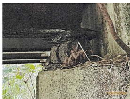
5 PHOTO - ROLLER BEARING CORROSION AT WAILUKU ABUTMENT NOT TO SCALE
