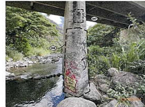
6 PHOTO - SPALLS / ABRASION ON PIER NOT TO SCALE
