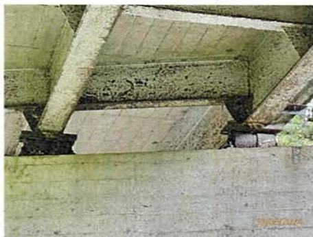
1 PHOTO - ROLLER BEARING CORROSION AT IAO PIER NOT TO SCALE
