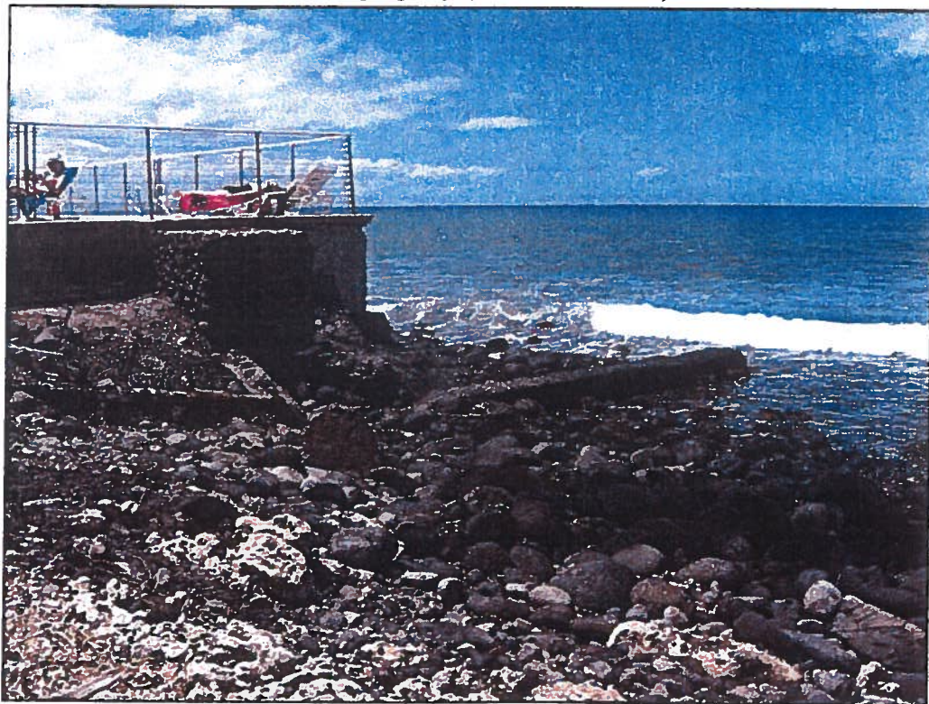
Photograph No. 2: Concrete groin at north side of swimming pool (Easement "E-2")
