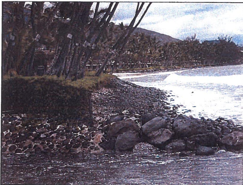
Photograph No. 4: View towards seawall encroachment south of the drainage channel (Easements "E-4" and "E-5")
