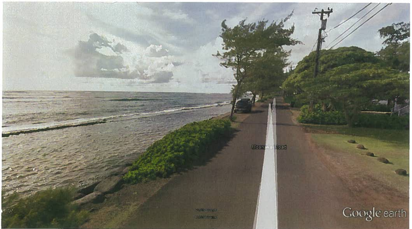
Topside- Southern reach with cap walkway in background; and Northern reach rubble rock mound in foreground
