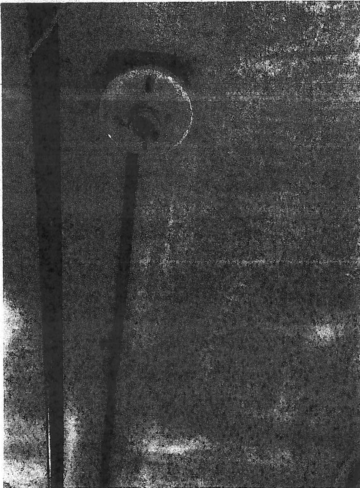
Exhibit V - ART 372.13 Discontinued outlets. Circuit conductors shall be removed from the raceway, Art 410.3 Live Parts. Luminaires shall have no live parts normally exposed to contact
