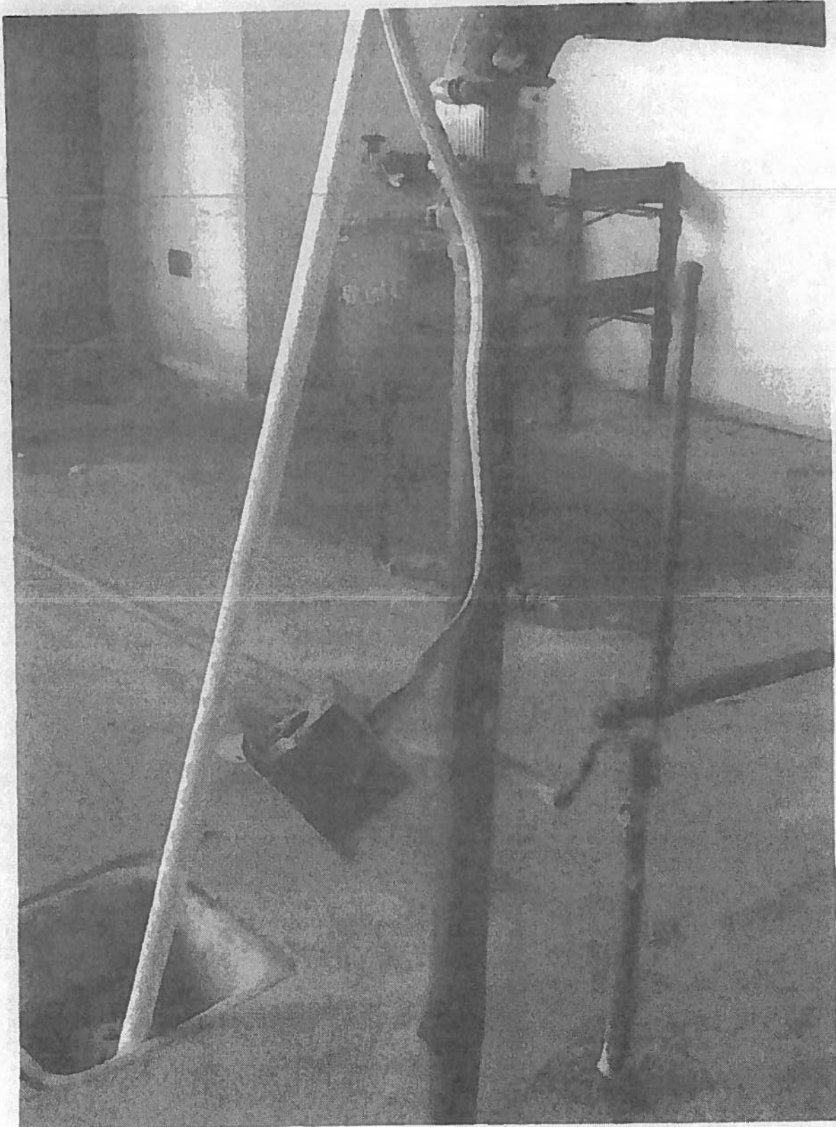
Exhibit P - ART 372.13 Discontinued outlets. Circuit conductors shall be removed from the raceway
