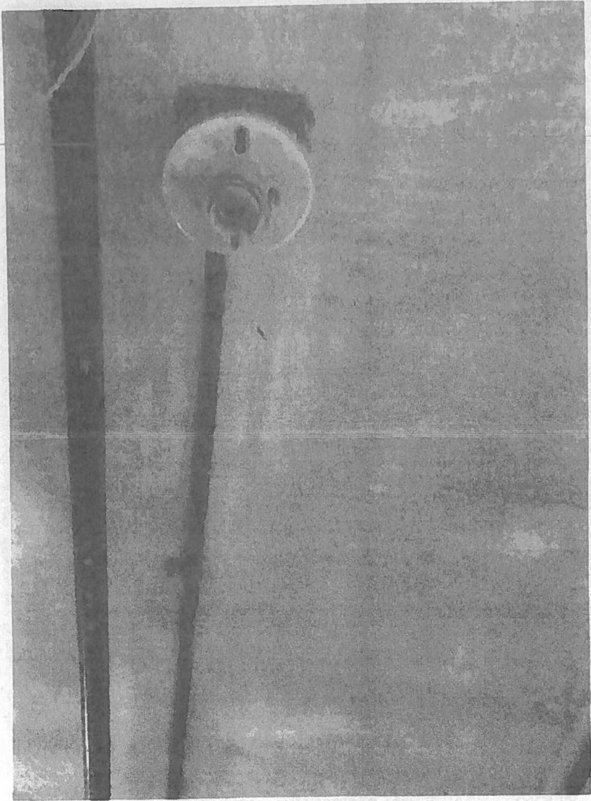
Exhibit V - ART 372.13 Discontinued outlets. Circuit conductors shall be removed from the raceway, Art 410.3 Live Parts. Luminaires shall have no live parts normally exposed to contact
