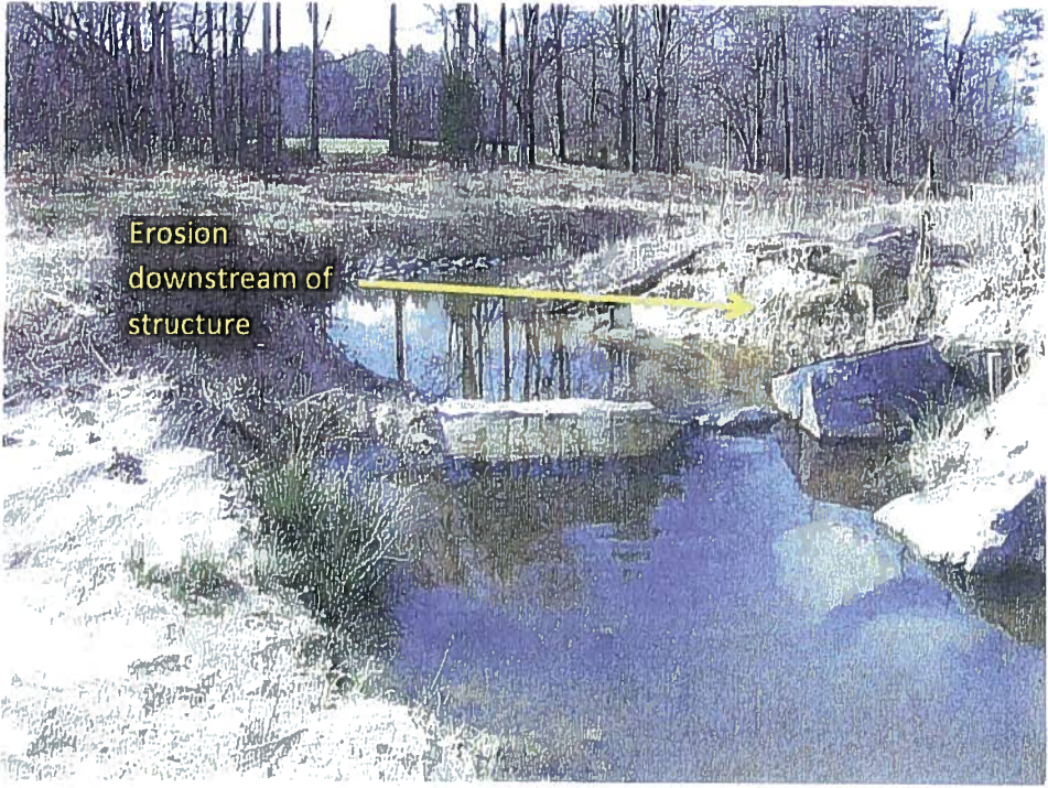
Photo 7- Erosion Downstream or Upstream of the Structure
