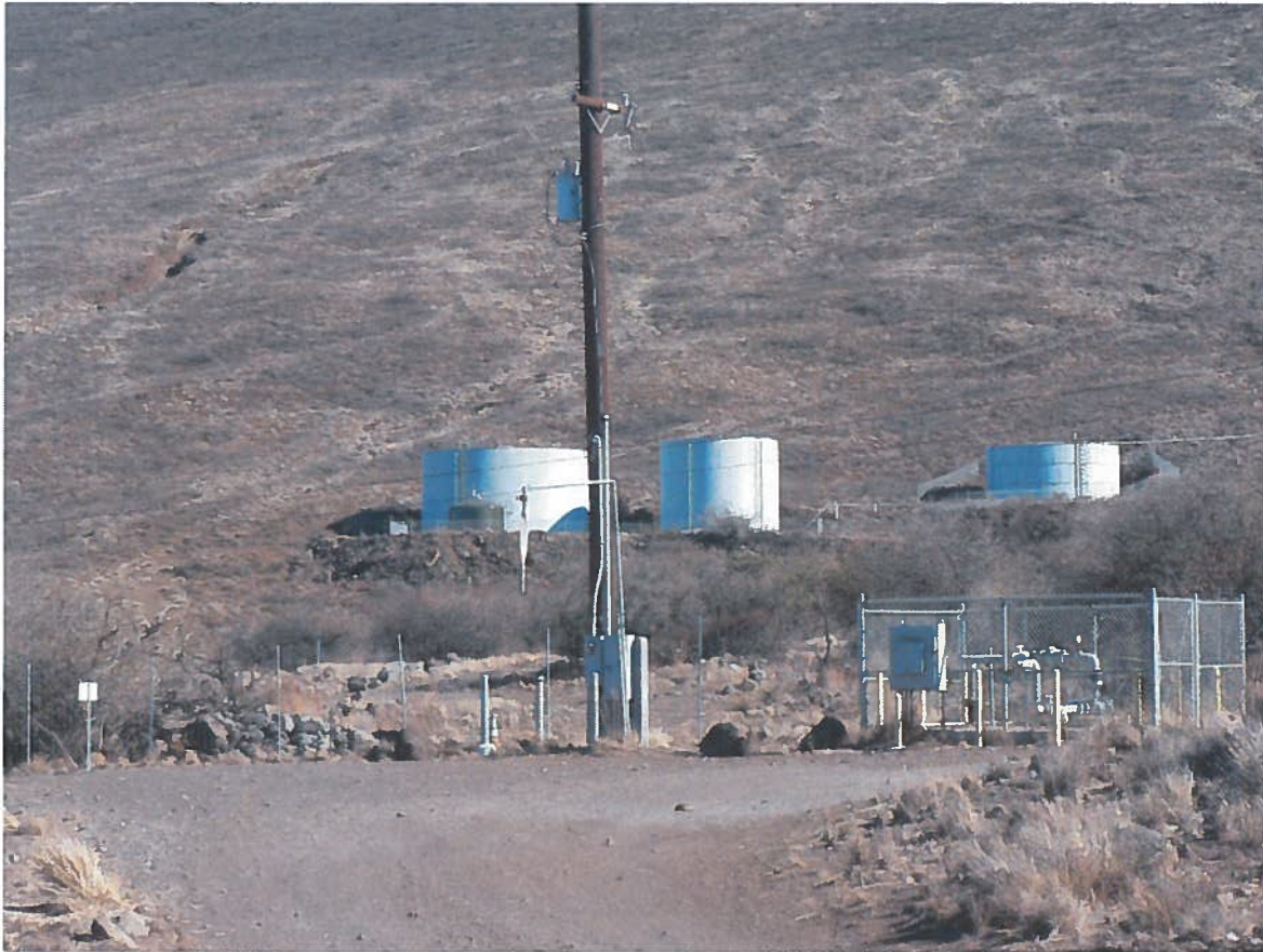
The water storage tanks of the water system
