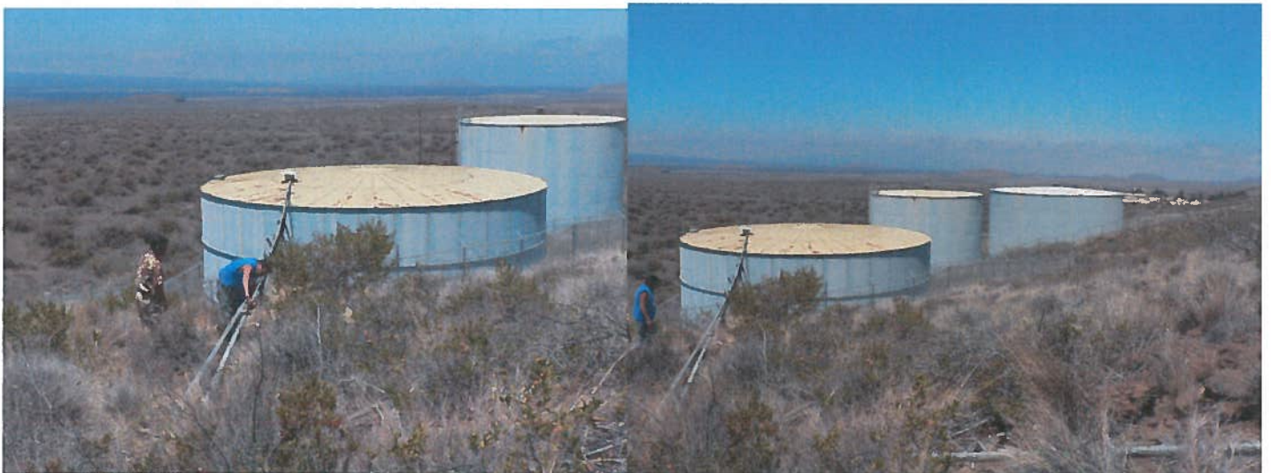
Photos of main feed storage tank and overflow tanks connected in sequence
