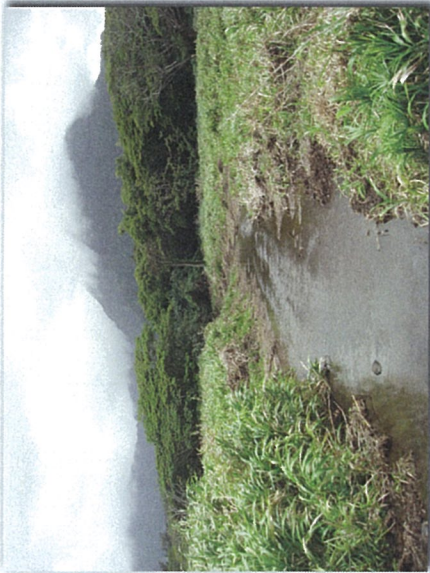
Photo 2: North view of Area A site conditions along Kapaa Quarry Road (near Le Jardin driveway).
