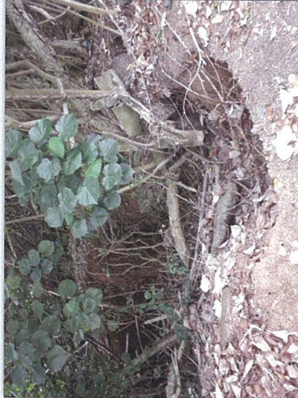
Photo 4: East view of Culvert 2 condition and erosion.
