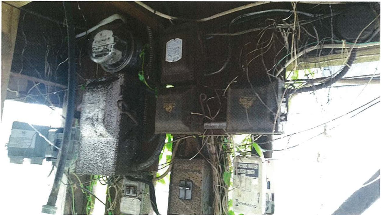
Main electrical panel and breaker box mounted under original house.
