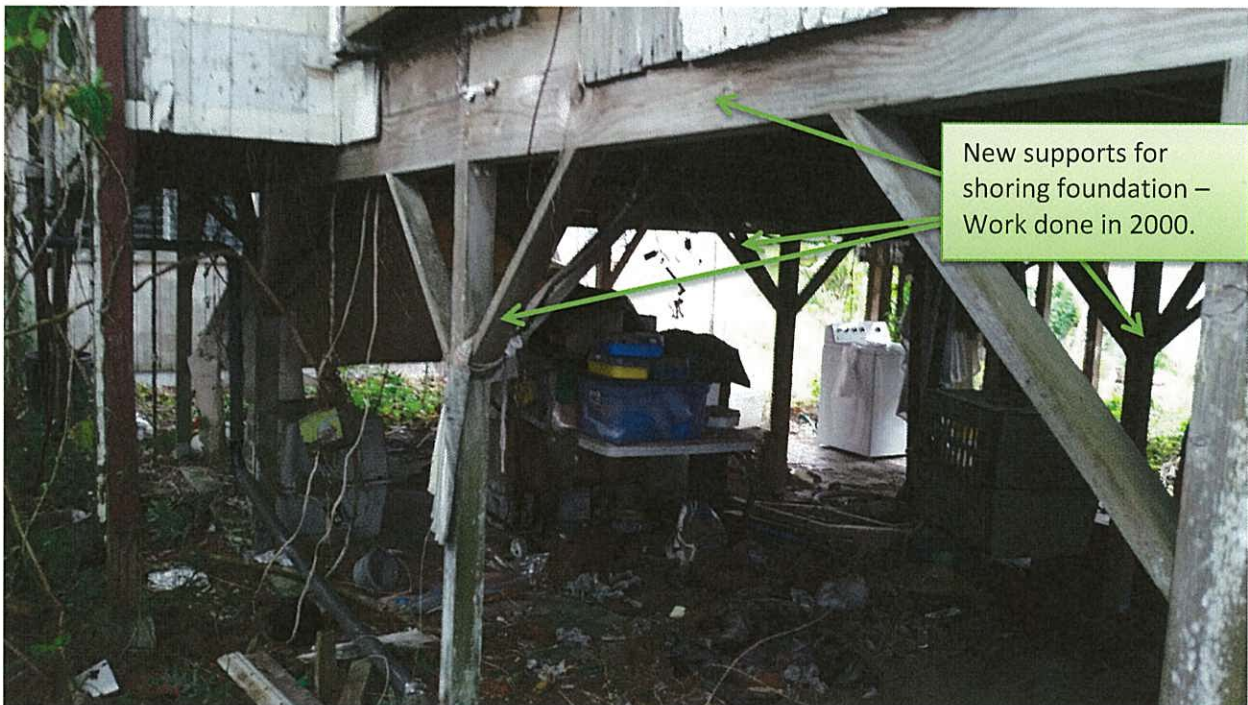
View of underneath of original house. The debris, wiring and vines are representative of overall condition of premises.
