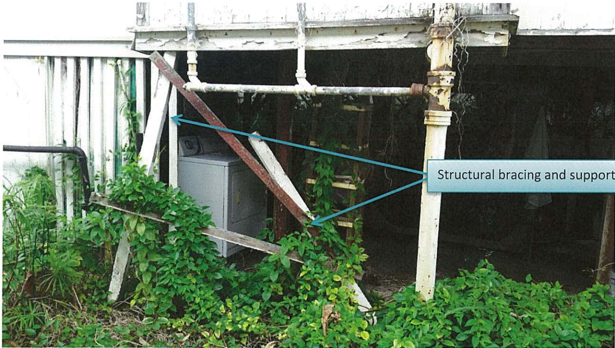
Side of original house. The support structure for the cantilevered bathroom has deteriorated leaving no bracing for that area of house.
