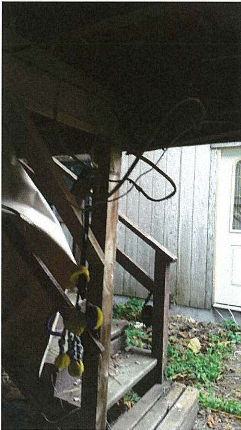
Electrical wiring and switches hanging under original house.
