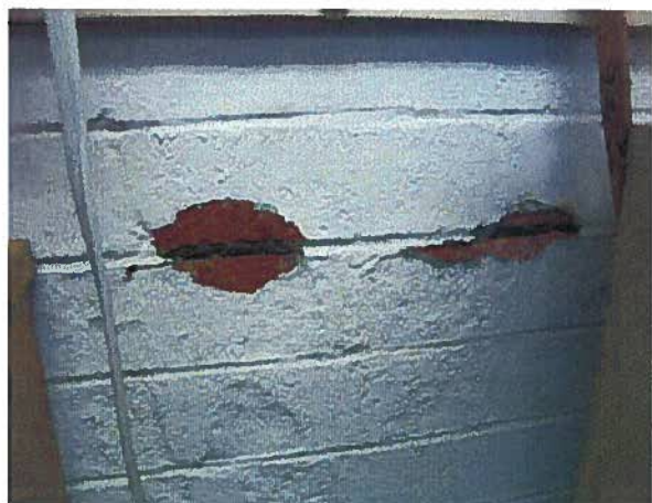
Photo #15 The photograph shows corrosion of joint reinforcing on the interior face of the masonry wall.
