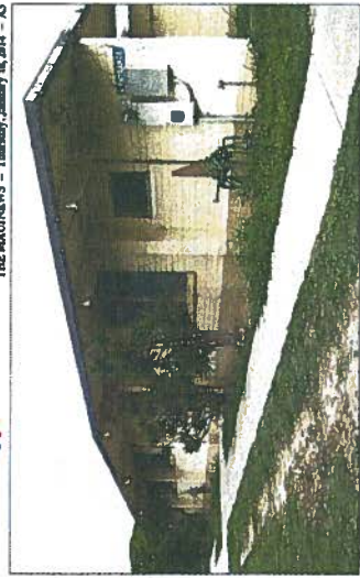
Originally built in 1989 as a juvenile detention center, the Department of Land and Natural Resources' Maui office in Wailuku was moved from several cracks and damaged in its structure over the years. The state department plans to replace the building with a $5.7 million administration building, according to plans for the preparation of a final environmental assessment.
