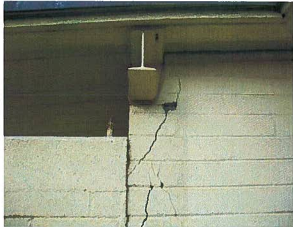
Photo #9 There are cracks in the masonry wall around the steel roof beam.
