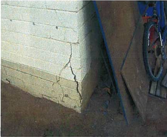
Photo #8 There are vertical cracks at the corner of the masonry wall.
