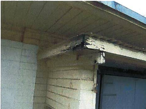
Photo #10 The roof framing for the existing attached storage enclosure has moisture damage.
