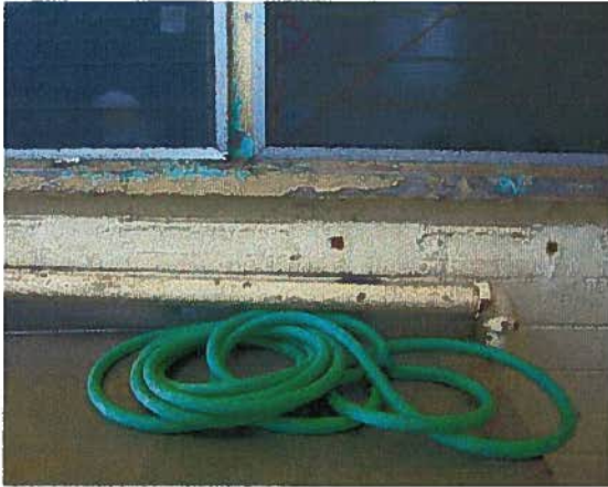
Photo #12 The photograph shows moisture damage and paint delamination at wooden window frames.
