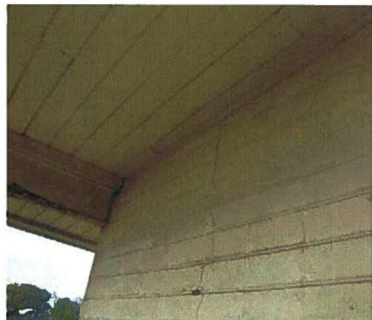
Photo #7 There is a vertical crack along the face of the masonry wall.
