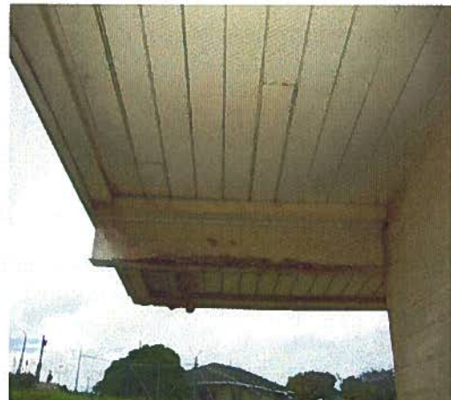
Photo #11 The bottom flange of the steel roof beam at an exterior eave has corroded.
