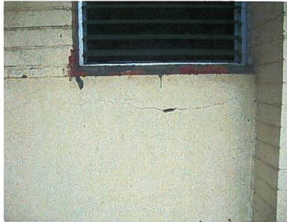
Photo #13 The existing cement skim coat finish has a surface crack.
