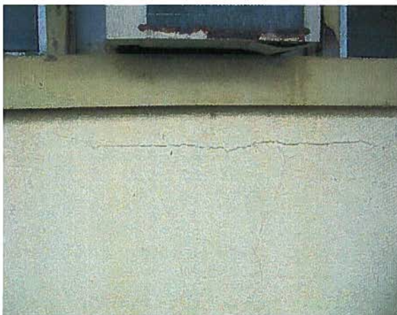
Photo #14 There is a surface crack in the existing cement skim coat finish.
