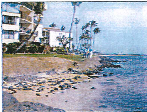
View of the sink hole behind the top of the existing seawall. Note small sand beach and base of Ma'alaea breakwall in the background.
