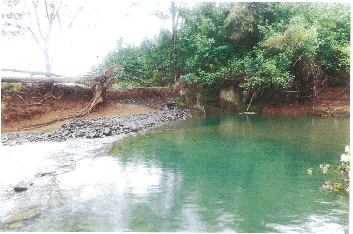
USFWS Intake Structure - After April 2018 Flooding
