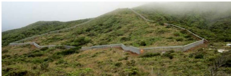
Enclosure A at the Makamaka'ole seabird mitigation site, West Maui, completed in May 2013.
