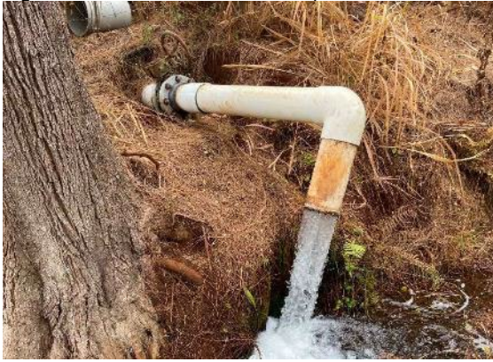
A) Water was originally released from a valved pipe from Reservoir 1 into the South Waikapū ‘Auwai, experiencing high amounts of water loss.
