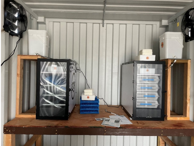
Photo 3. Cabinet incubator and hatcher in the EH Wildlife programs hatching/brooding facility. Electrical and ventilation were installed during FY24 using WLR.
