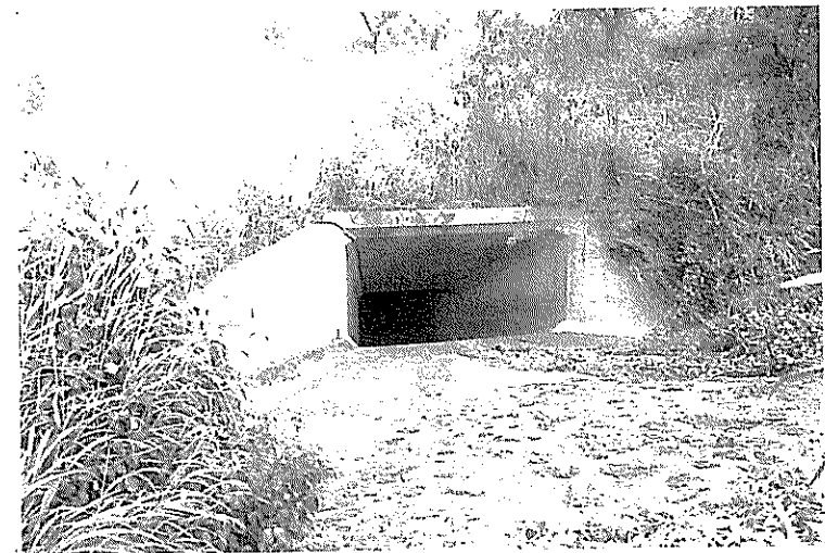
Figure 4. Top: Overview of Parcel 64, View to North. Bottom: Concrete Culvert, View to North.
