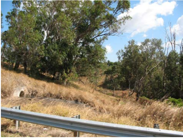
13. View of a drainage wall observed along the northern portion of the subject property.
