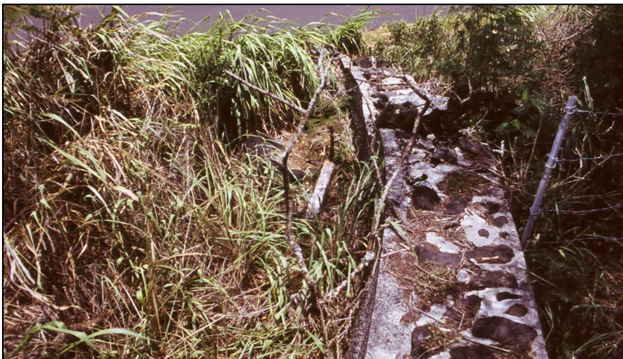
Figure 15. View of concrete irrigation culvert at edge of Hapa Road. View to east.
