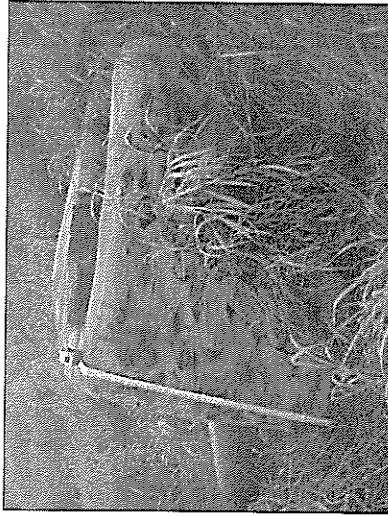
Figure 43. Feature G basin, showing steel pipe extending downslope to Honouliuli Stream, view to the south
