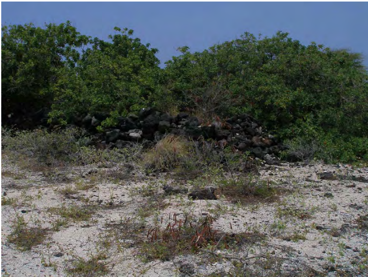
Figure 30. SIHP Site 1911 southeastern corner of enclosure documenting current state of wall collapse.
